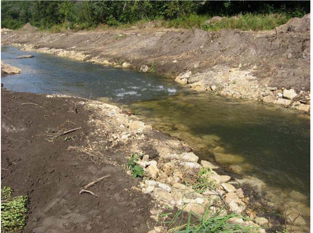
Progress on 6 September 2008. Top: A new weir. Bottom: View of the downstream reach before grading.
